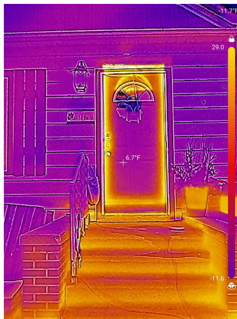
Figure 9. A thermal image of Resident #2's front steps and door There is a temperature scale on the bottom with -11.6 Fahrenheit being the lowest (purple) and 29.0 Fahrenheit being the highest (yellow-white). The frame of the front door is a warm yellow while the door itself and the main house is a pink-purple.
