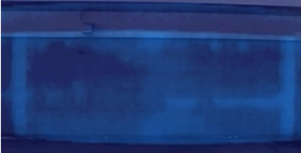
Figure 3: A thermal image taken by the drone of the back wall of the Morris City Hall The thermal image shows lower temperatures in darker blues and higher temperatures in lighter blues. The interior office partitions are visible in light blue on the left and right of the image. The ceiling is also visible in light blue.
